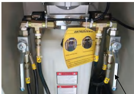
Oil Filling Position
